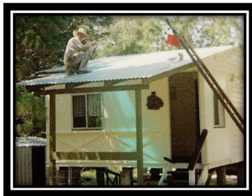
Photo 3: Noel working on the first stage of renovations, replacing and expanding the roof
